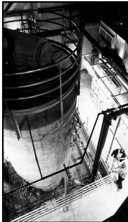
Juneau's new sewage sludge incinerator.
